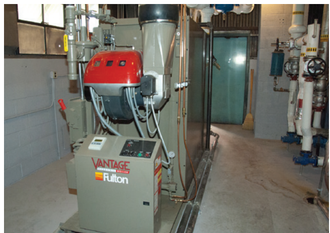
Vantage Hydronic boiler for the District 9 office.
