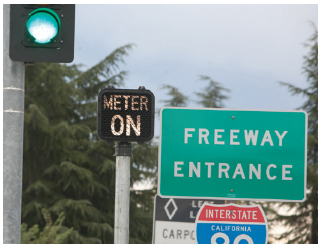
Freeway ramp meter indicator.
